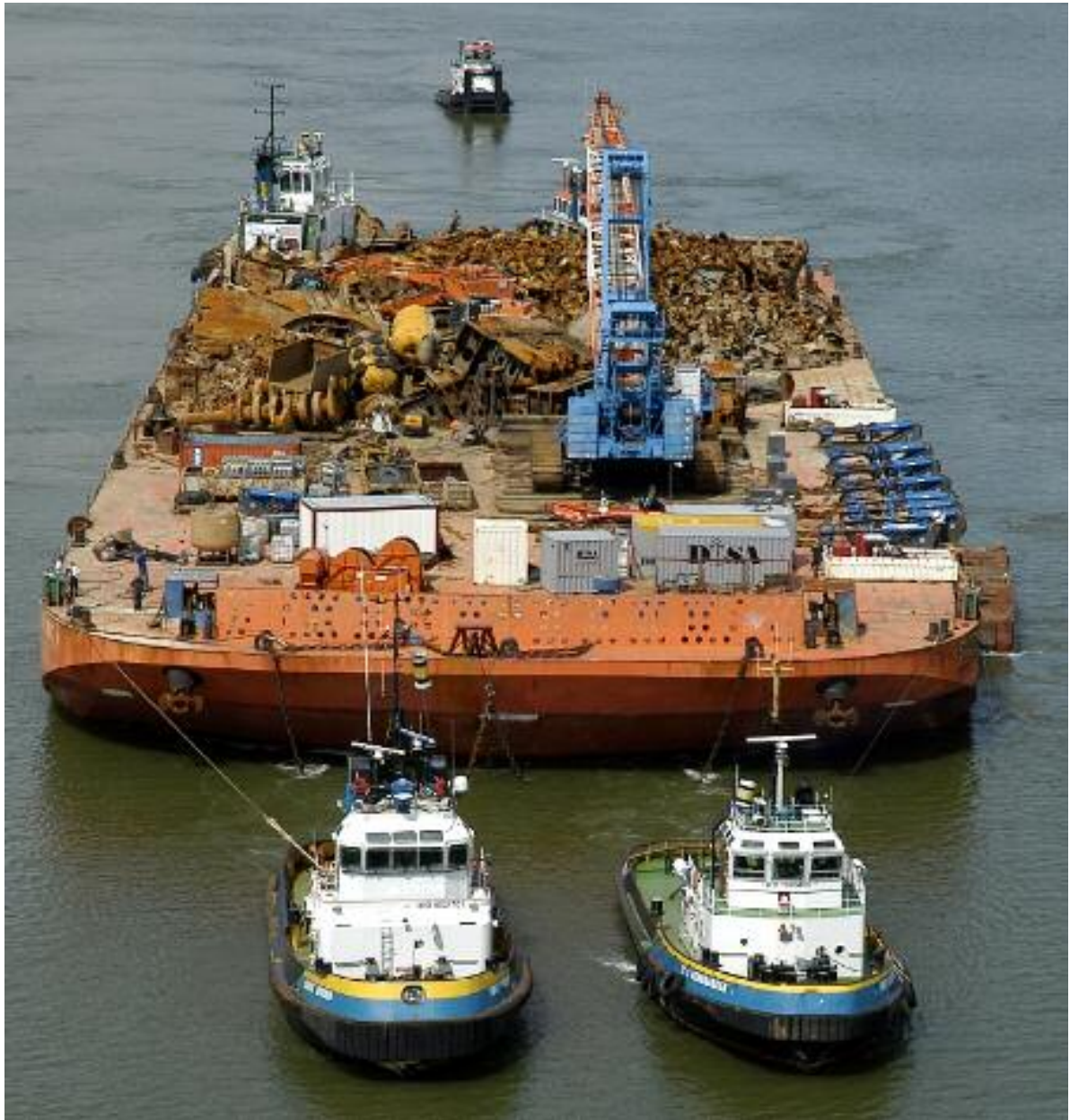
Above seen the last barge, SAINTY No 8 with onboard the chain pullers and the last scrap (including the crankshaft) of the MSC NAPOLI , passing the Botlekbridge in Rotterdam enroute from Lymebay to Dordrecht
