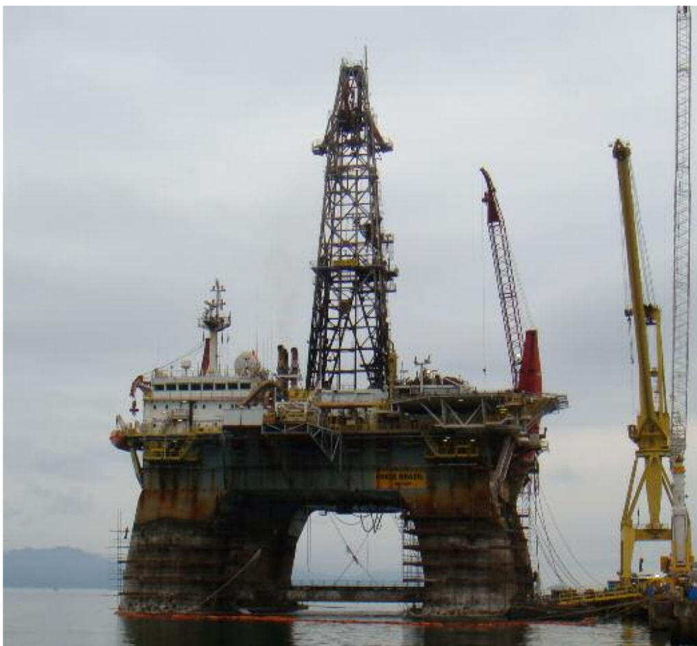
The rig Pride Brazil seen above at Angra dos Reis in Brazil during repairs at the Keppel yard Photo : René Guerra ©
