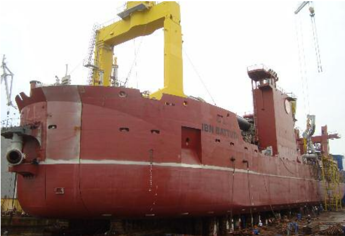
The first of a series of 4 self propelled cutterdredgers under construction at the Uljanik shipyard in Pula (Croatia) for Jan de Nul is named IBN BUTTATA was launched August 14 th
