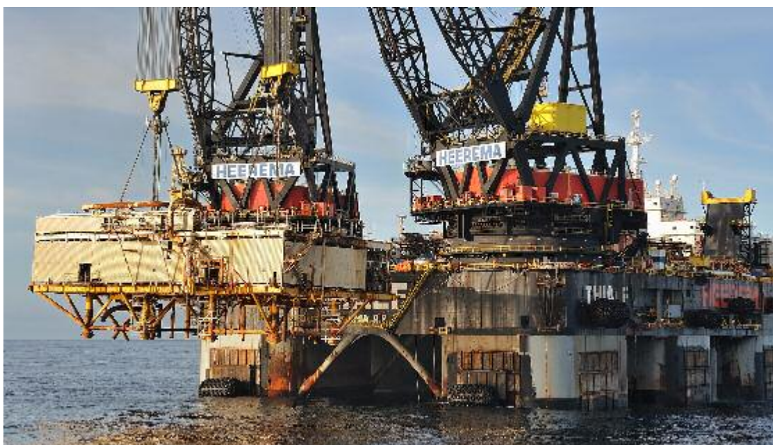
Heerema's Thialf seen removing the Ekofisk 2/4R module Photo : capt Jan Berghuis – Master Retriever (c)
